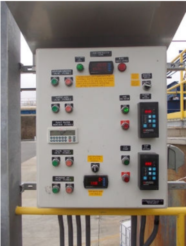
Figure 2: Power Sensors in action in a Water Treatment facility
